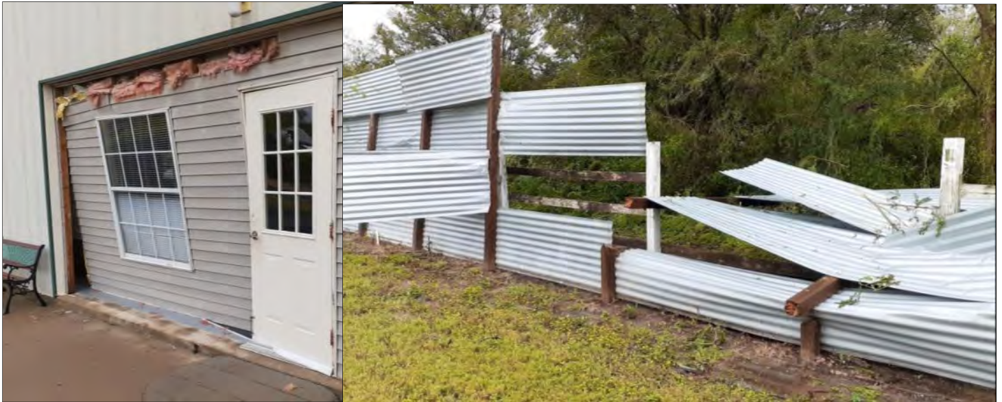
Damage from Hurricane Hanna
