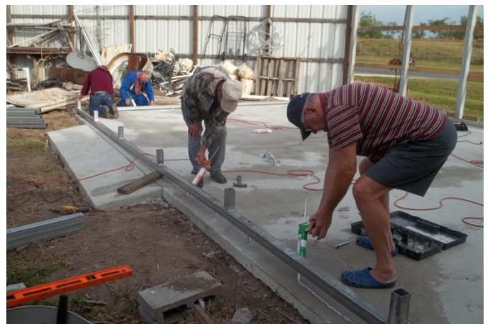
Our team of Volunteers waterproofing the base of the new Storage Shed
