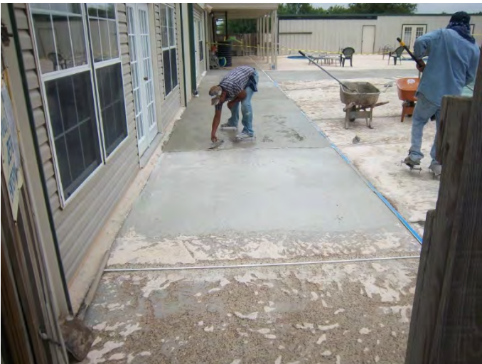
The Cool Deck has been chiseled off, and the Leveling Layer is being applied.
